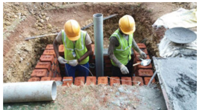
Rainwater harvesting pit owned by STT GDC India
